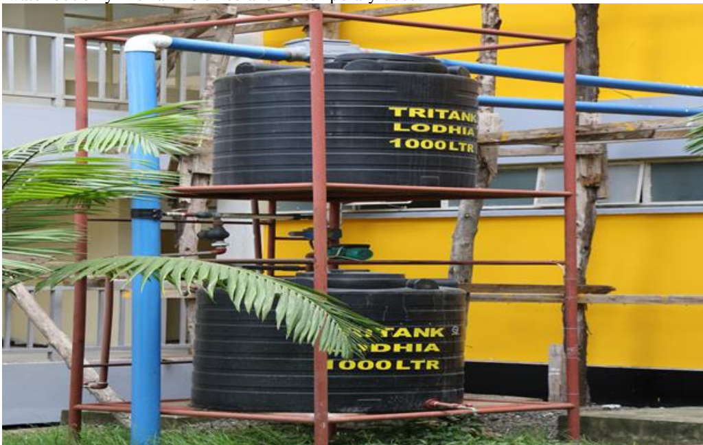
Figure2. RWH using small tanks at ATC, Project at water quality unit,
