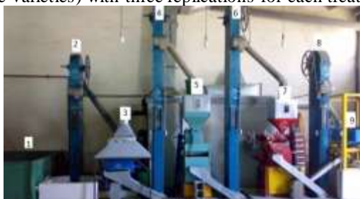
Fig. 1. Main components of a typical milling system used in Iran's rice mills
