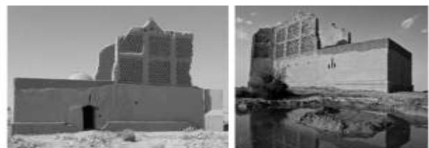
Figure 12. Set-backs and juts of east and west wall, which add to the beauty of the structure
