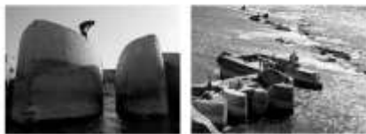
Figure 17. The outer view of the ship foundation which is caulked with gypsum and mortar and filled with mortar
