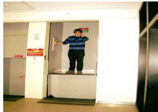
(c) Paternoster located in a office building
