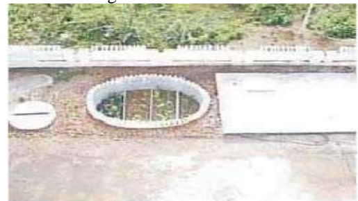
Fig.8 Root Zone Treatment bed
