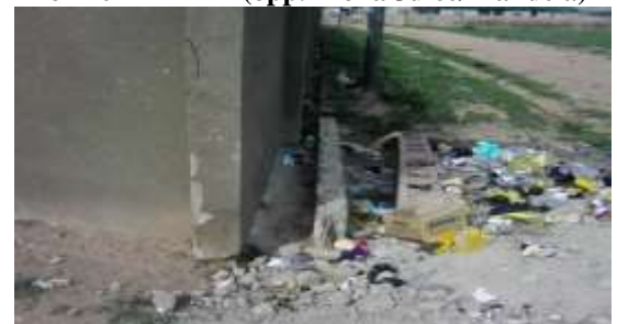
Plate III: A collapsed drainage network at MTP 3 (Morris Fertilizer)
