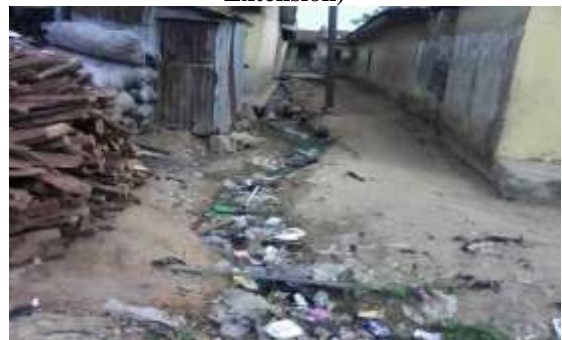
Plate II: A drainage network filled with dirt and litters at former MTP 47 (opp. Mona Juice/Mandela)
