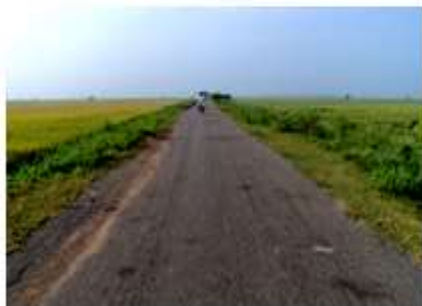
Figure 2. View of Rural Road Surface damaged Palem - Kollimerla (G1) in Guntur District.
