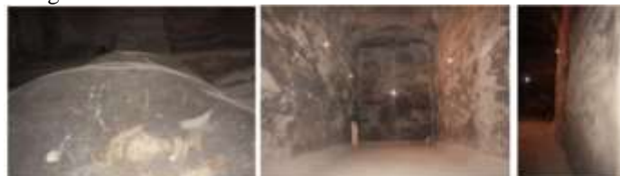
Fig 3. Interior space of reservoir- Untidy projected volume (Tableh) on Reservoir wall
