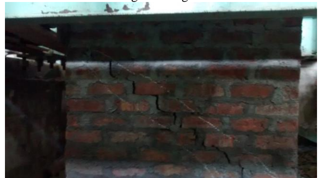
Figure 2 crack pattern in simple masonry
