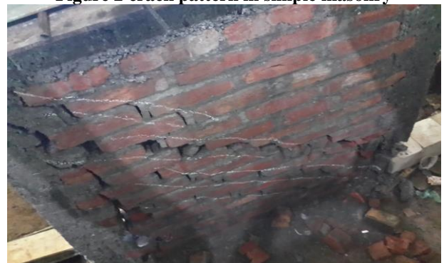
Figure 3 crack pattern in confined masonry
