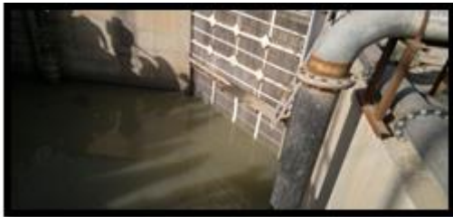
Fig 4. Bar Screen of RWTP
