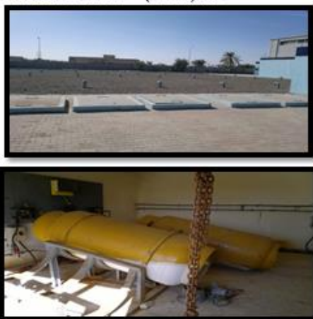
Fig 8. Ground reservoir and Chlorine Container of RWTP Data Collection
