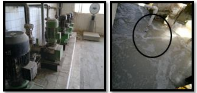
Fig 5. Rapid Mixing and room of alum add in RWTP
