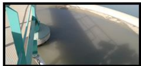
Fig 6. Sedimentation basin with scraper in RWTP
