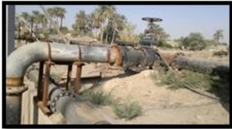
Fig 3. River Intake and Main pipe of RWTP
