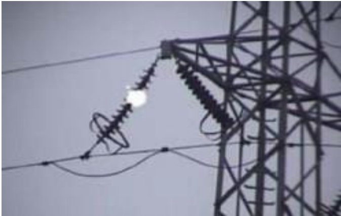
Fig 1. Visible Corona Effect in transmission line
