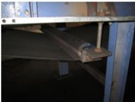
Photograph 3.3. Use of return idler to increase belt tension
