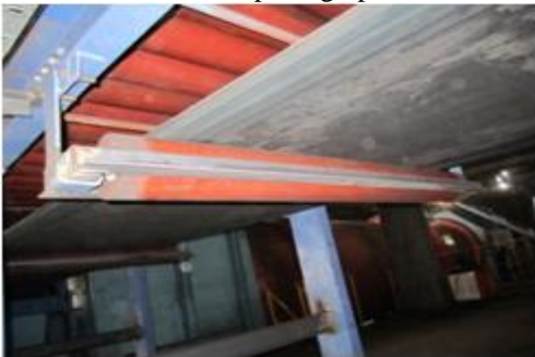
Photograph 3.2. Brackets for return idler
