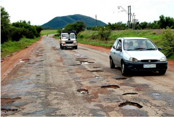
Figure 3. Damage to roads due to heavy freight transport. Objective
