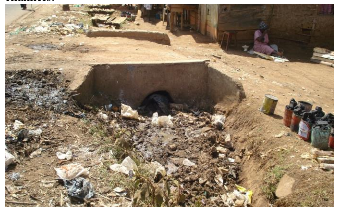
A photo showing storm drainage channels which have been rendered dysfunctional due to lack of regular servicing.
