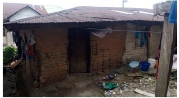
Figure 5. Mud Building with Rusted Corrugated Roof.
