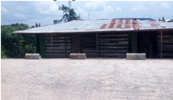
Figure 2. Wooden Building with Rusted Corrugated Roof.
