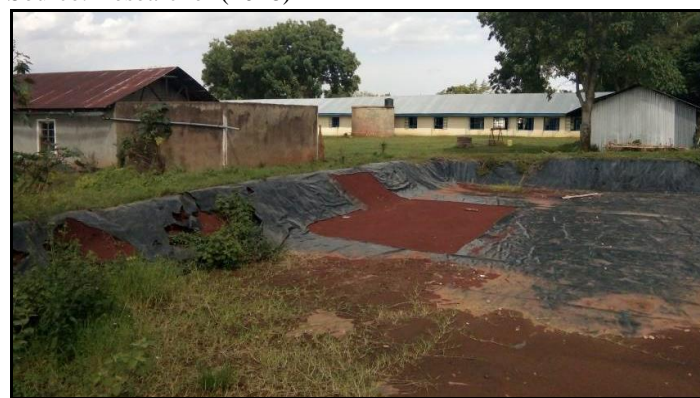
Plate 3. A neglected PVC-lined fishpond at Luanda Dudi Secondary School in Khwisero Sub-county, Kakamega County, Kenya
